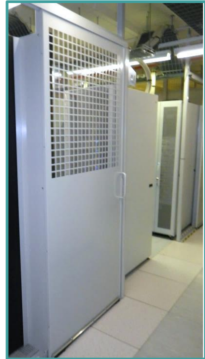
Fig. 6: image of aisle containment
