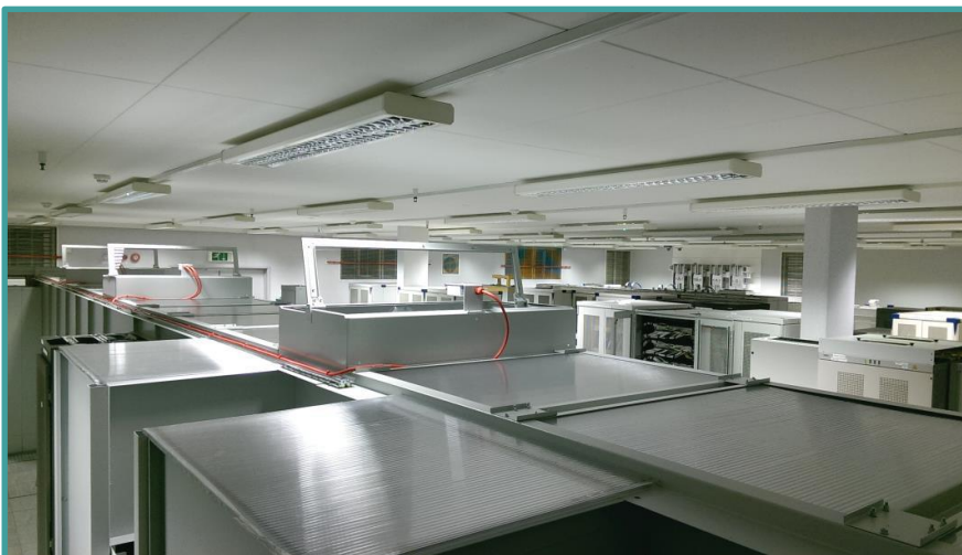
Fig. 7: image of roofing system for aisle containment
